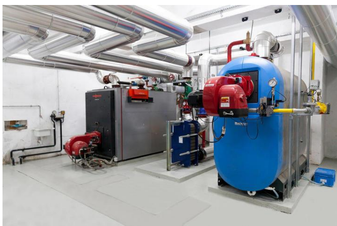
Picture 40.: The renovated boiler room in Deteljica Source: https://www.finance.si/
