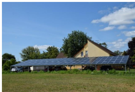
Picture 36: Zahony Municipal Buildings, PV panels
