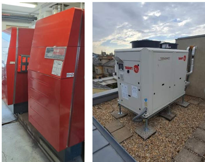
Picture 22: New gas boiler and central cooling system @ Árpád Petrovszky, condominium manager
