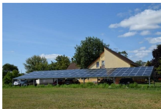
Picture 36: Záhony Municipal Buildings, PV panels.
