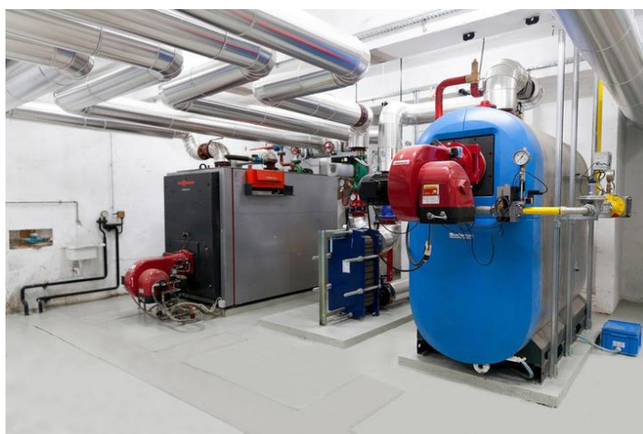
Picture 40: The renovated boiler room in Deteljica, source: https://www.finance.si/okolje-energija/%28video%29-z-energetsko-prenovo-do-pol-milijona-prihrankov/a/8947028
