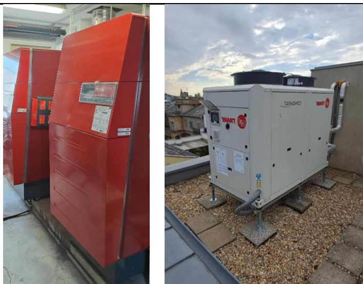
Picture 21: New gas boiler and central cooling system.
