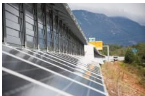
Picture 43: The PV panels on Bazara, source: https://sempeter-vrtobja.si/postavitev-soncne-elektrarne-na-protihrupni-ogradi-hitre-ceste-pri-bazari-svicarski-prispevek/highway
