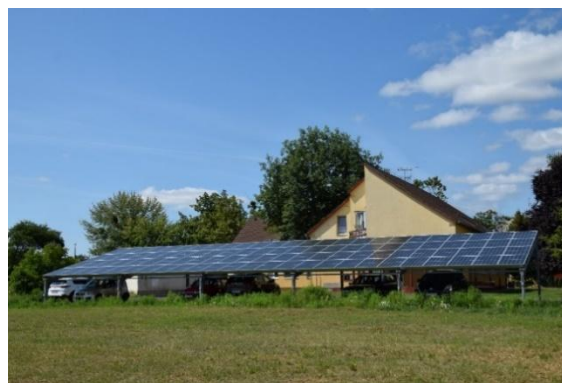
Picture 36: Zahony Municipal Buildings, PV panels
